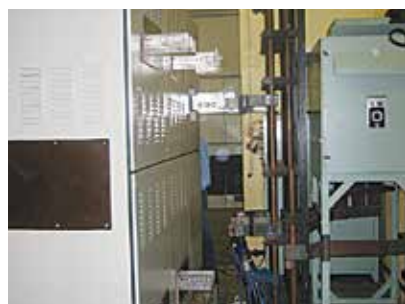
Short Circuit Test
