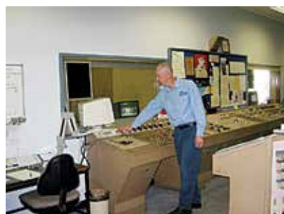
Short Circuit Test from Control room
