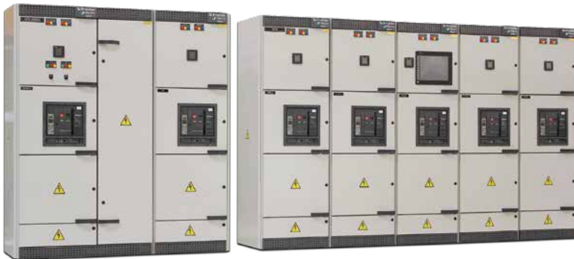
Main LV Switchboards
